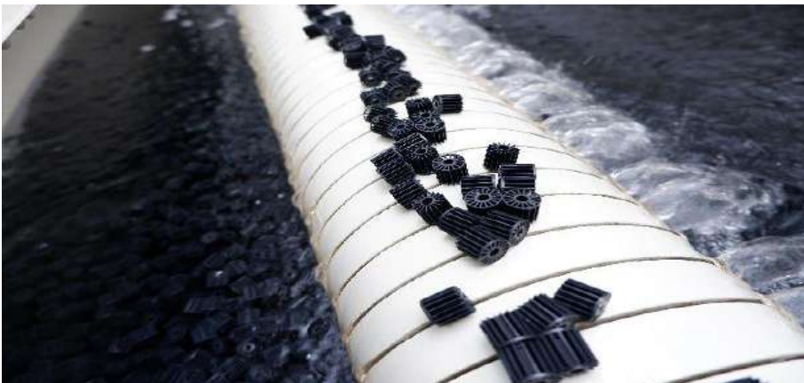
Figure 8. Moving bed bioreactor and media inside.
