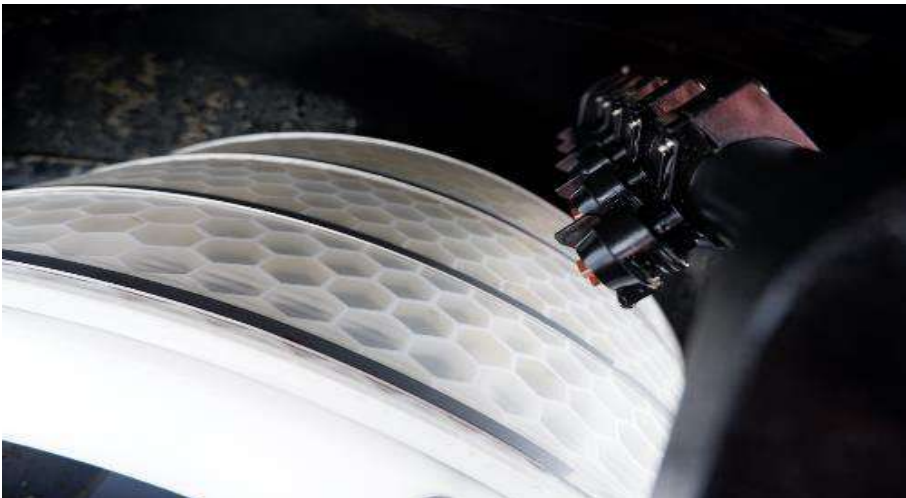
Figure 7. Inside view of a drum filter and backwash mechanism.
