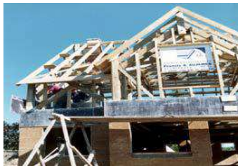
Figure 9. View of the building constructed with industrial hemp building material located in France [36]
